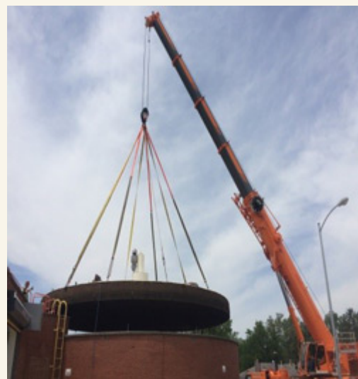
PSC Lifting a 70,000 lb. Digester Lid at a local Waste Water Treatment Plant
